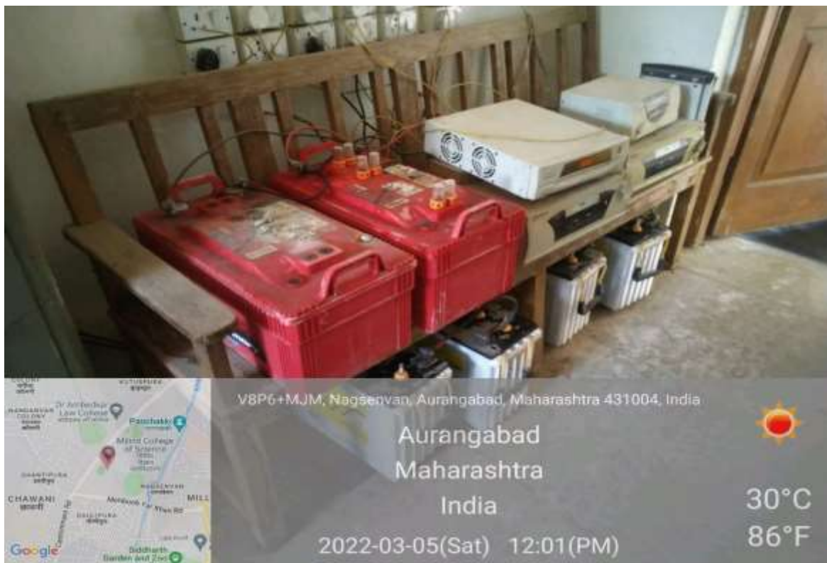
Inverter batteries used in the campus
